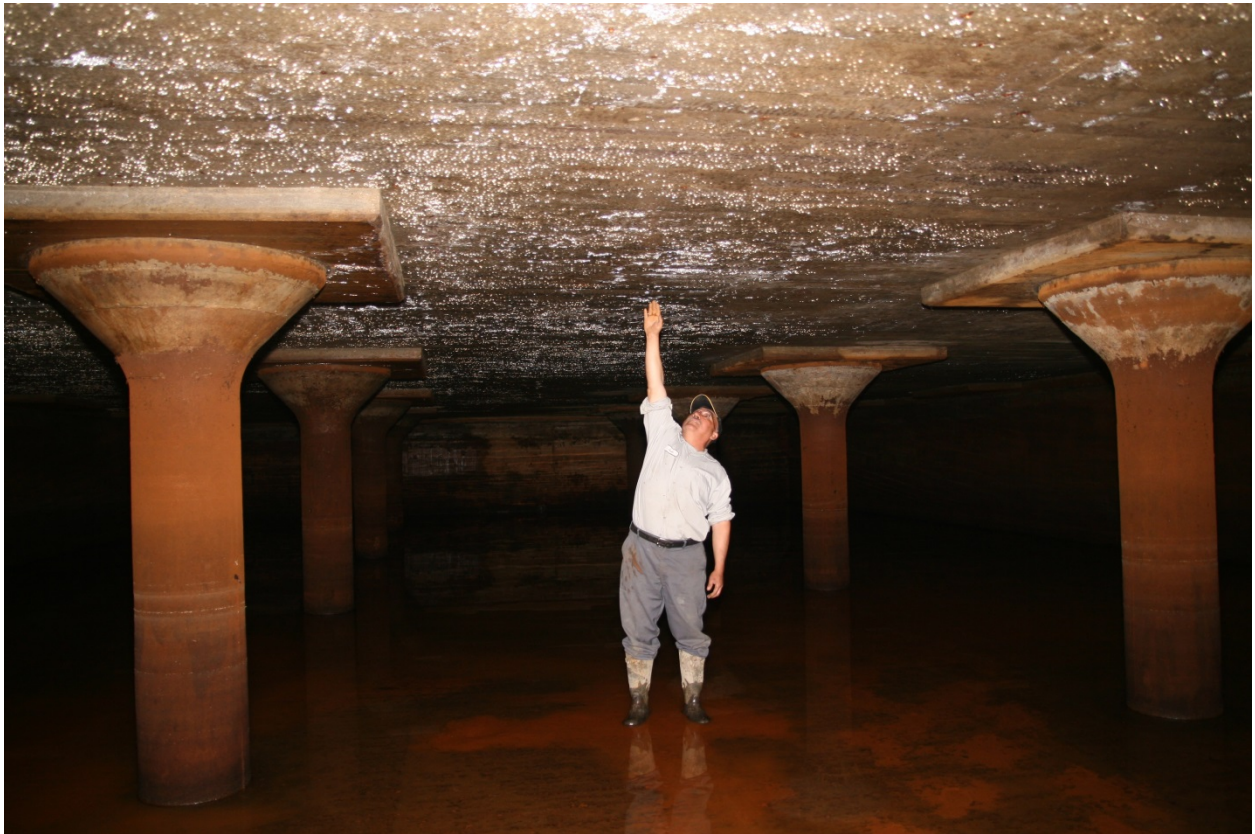
Underground tank dimensions are 115' x 50' x 11' tall which holds 473,000 gallons of water.
