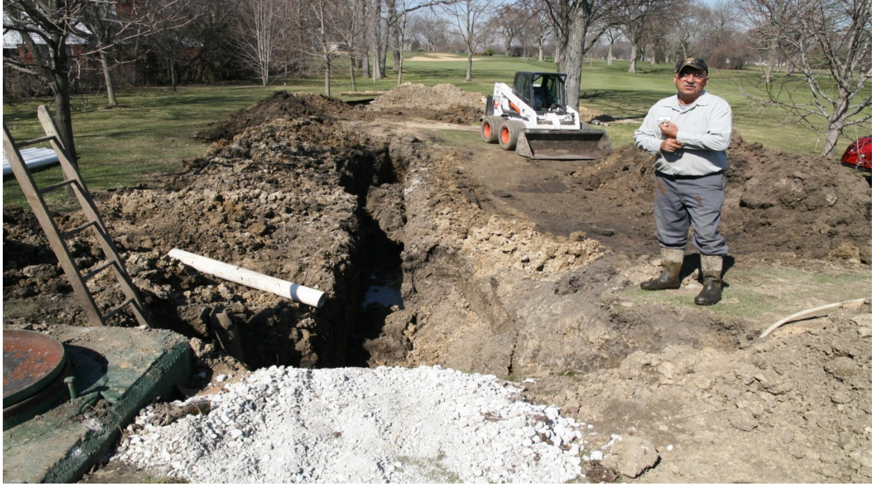
Some modification was necessary to valve off line that drains into pond. All work was done in-house.
