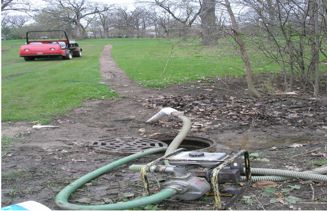
Pump used to move storm water from manhole into underground line that feeds into storage tank.
