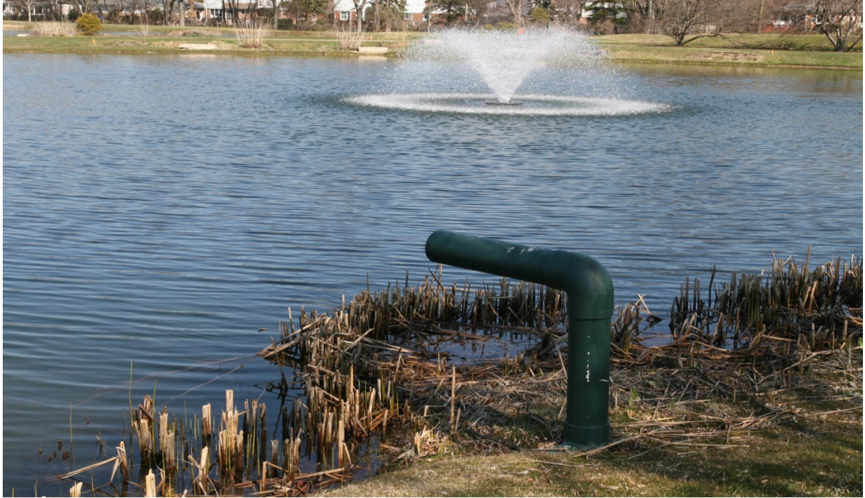
The outlet into the pond has an air gap to ensure no back siphoning.
