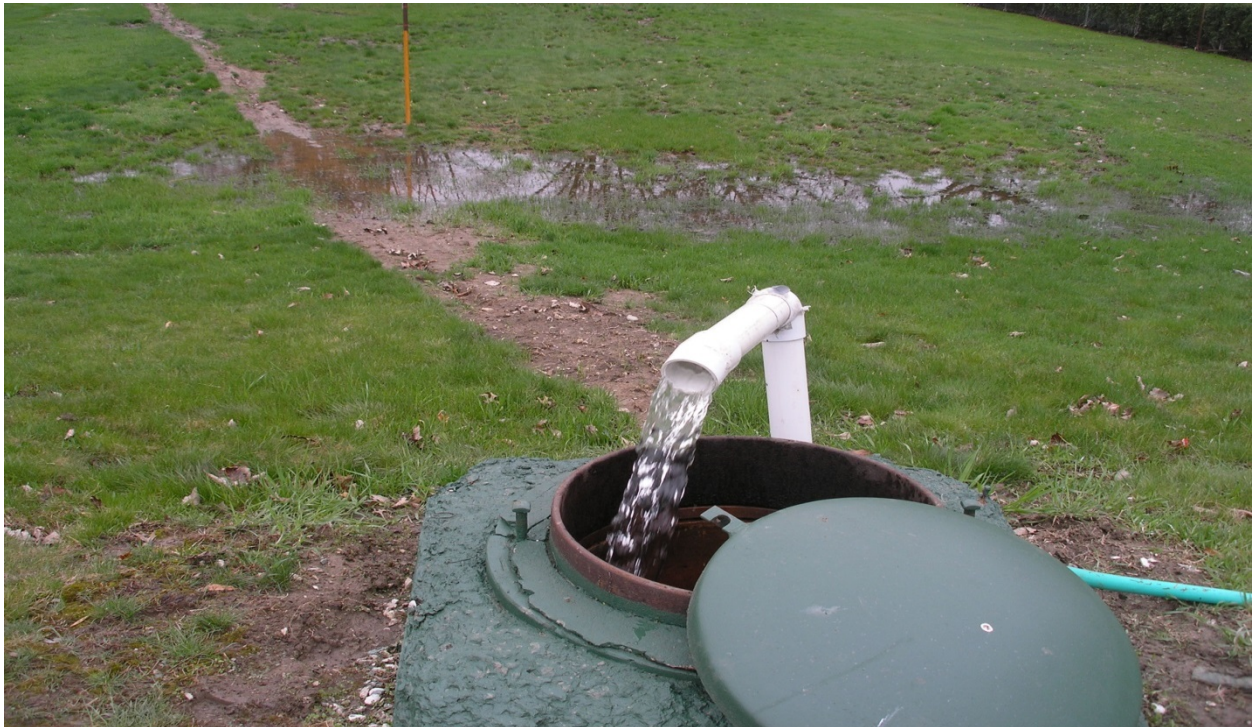
Outlet filling storage tank is a 'waterfall' design to help aerate water during fill.
