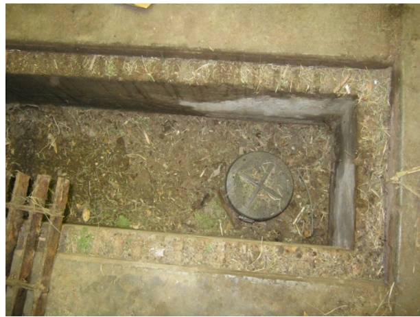
Open drain plugged to safeguard environment.
