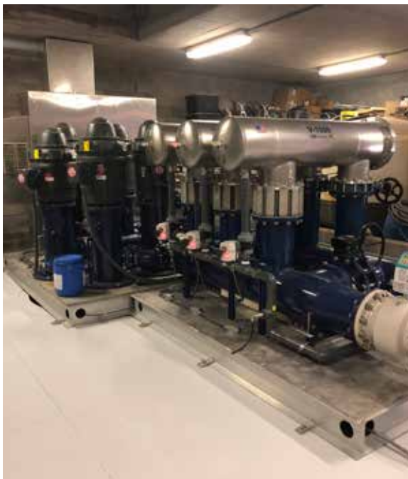
Kohanaiki Pump Station
