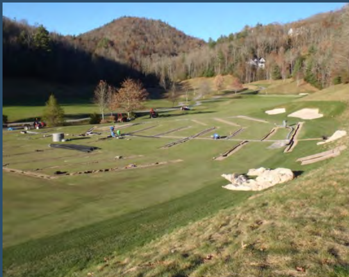
Extensive drainage improvements may need to be done in phases, so proper planning is essential.
