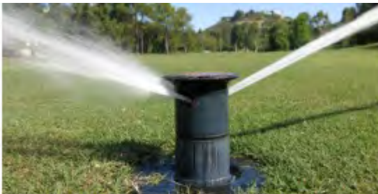
Sprinklers should be checked every week to ensure that they properly pop up, turn, and retract. Check that they rotate at the correct speed and that they are not leaking.
