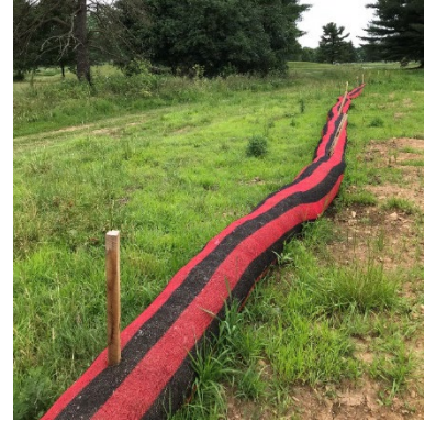
Figure 1. Erosion and sediment control is a critical aspect of all construction activities when soil is disturbed.
