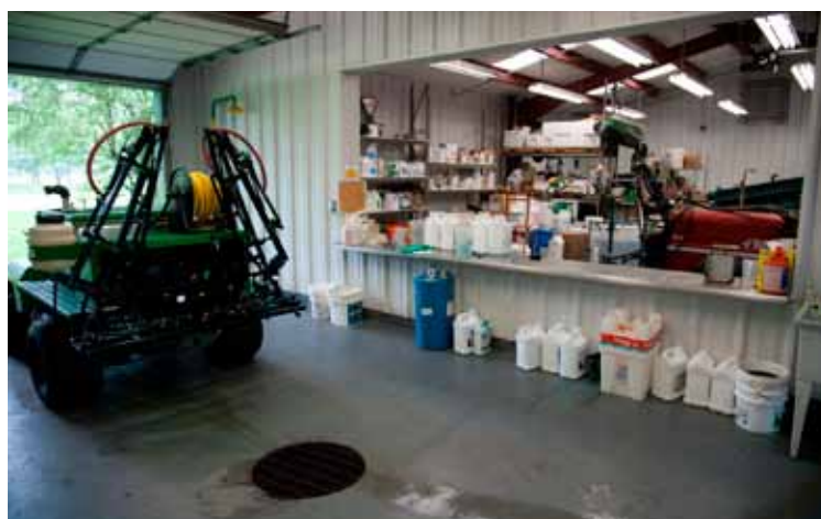
GCSAA recommends that mixing and loading areas have several safety features including an impervious floor capable of containing liquid spills with overhead protection from the weather. Photo © Montana Pritchard
