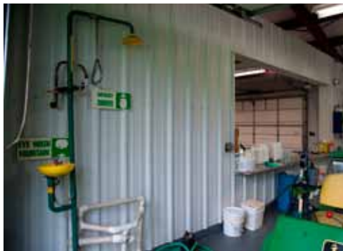
Pesticide storage and mixing/loading areas should have an emergency shower or eyewash station nearby. Photo © Montana Pritchard
